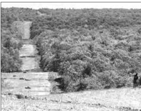
After construction on the Tennessee Gas Pipeline right of way in West Milford.
